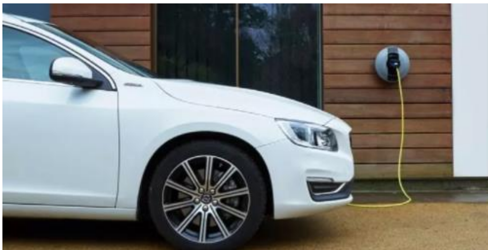
Figure 8. Residential charging point
